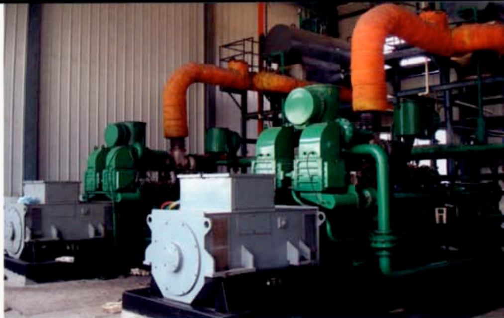
Methane power generating units at the Pingdingshan mine in Henan Province, China. The mine captures and uses 100,000 metric tons of methane per year.
